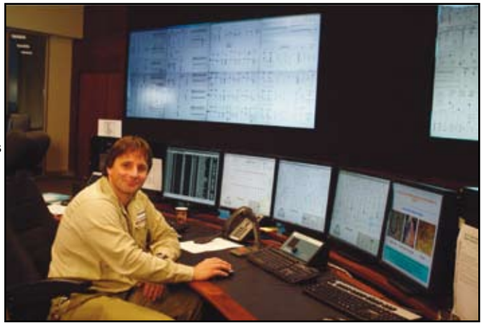
Figure 3. Modern control room with ergonomic desktop and overview displays.
